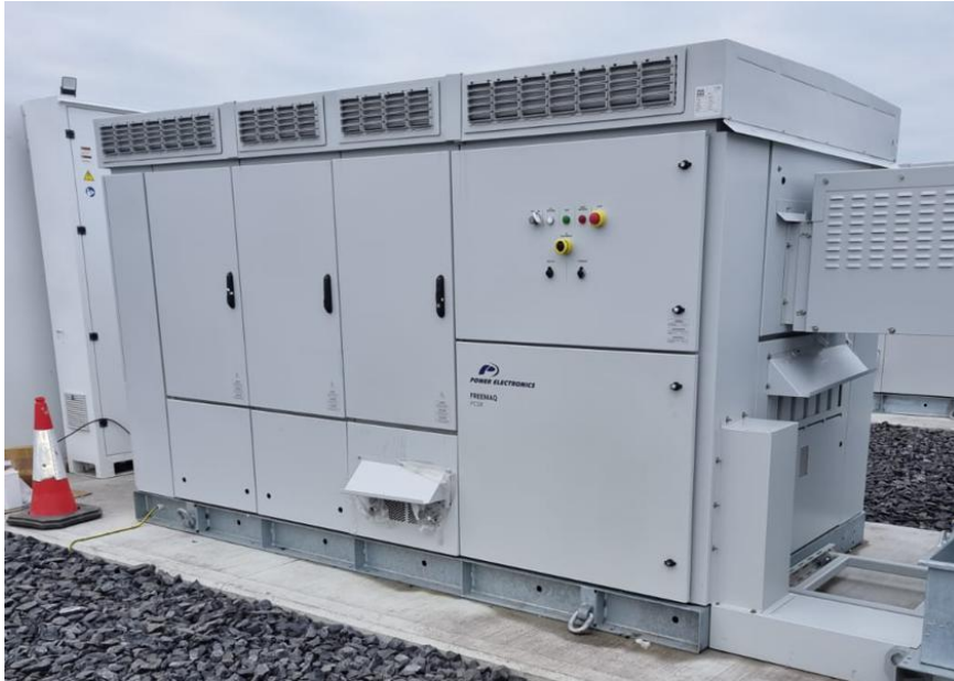
Figure 3: Fluence TX Inverter Station
